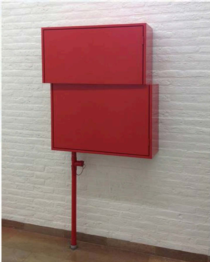
Roeland Tweelinckx, 'Fire hose cabinet (intervention)', variable dimensions, 2016
